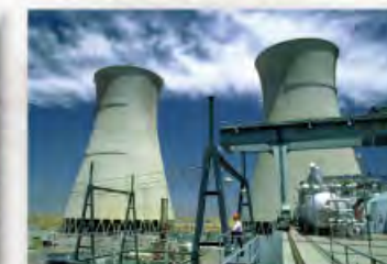
110kV Substation of Baiyinhua Third Mine of CPI Mengdong Energy Group Co., Ltd.
