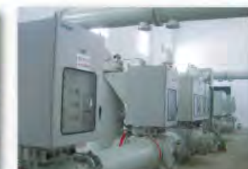
Yilan Wuguocheng Substation of Heilongjiang Electric Power Company
