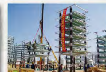
Jining Yinhe Substation of Shandong Electric Power Company
