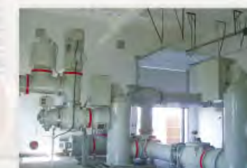
Qinhuangdao Nanlizhuang 110kV Substation engineering of North China Power Grid
